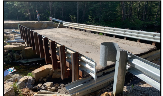
Above: Damaged bridge; Credit: Kathryn Emmitt
