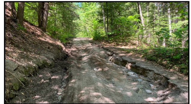
Below: Road washout; Credit: Kathryn Emmitt
