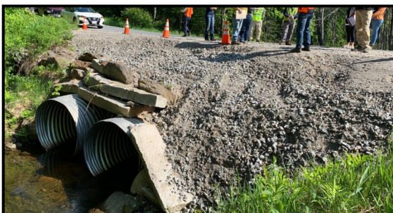
Washout around culvert; Credit: Kathryn Emmitt
